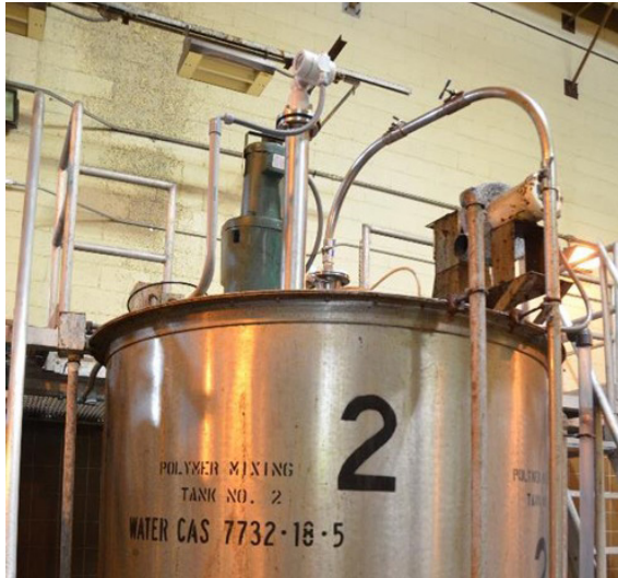
Polymer Mixing Tank
