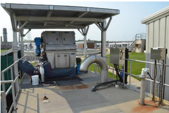
Bar Screen at TTO Pump Station
