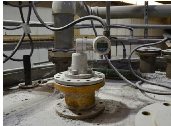
ABB LLT100 on Top of Sludge Storage Silo
