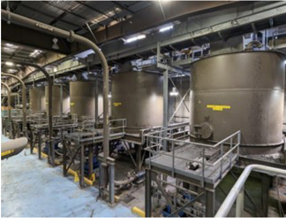
Five Sludge Storage Silos
